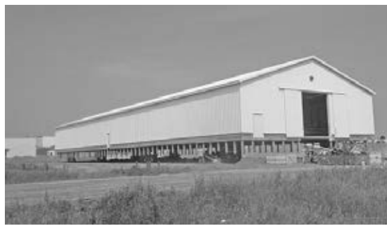
Need to move or hold up a barn, pole barn, silo, house, or anything over size or weight? We have the equipment, personnel, experience & insurance. (616) 836-1911
